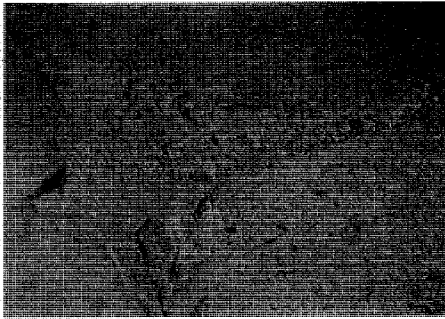
FIG. X2.47 High-Severity Spalling, Corner
