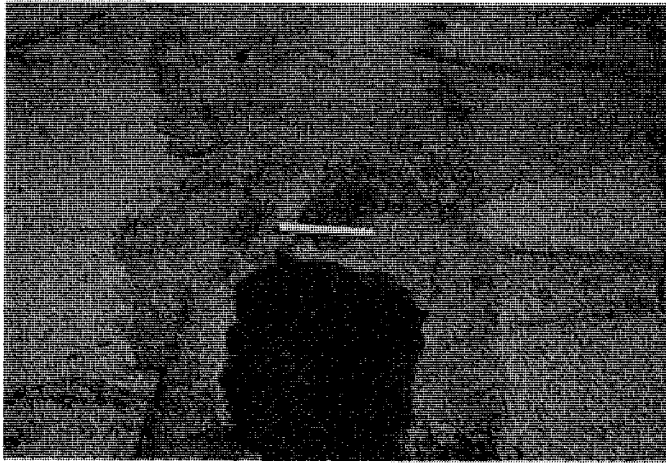
FIG. X1.33 High-Severity Patching and Utility Cut Patching
