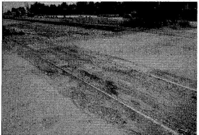
FIG. X1.40 High-Severity Railroad Crossing
