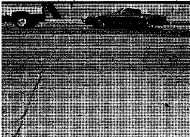
FIG. X2.48 Low-Severity Spalling, Joint
