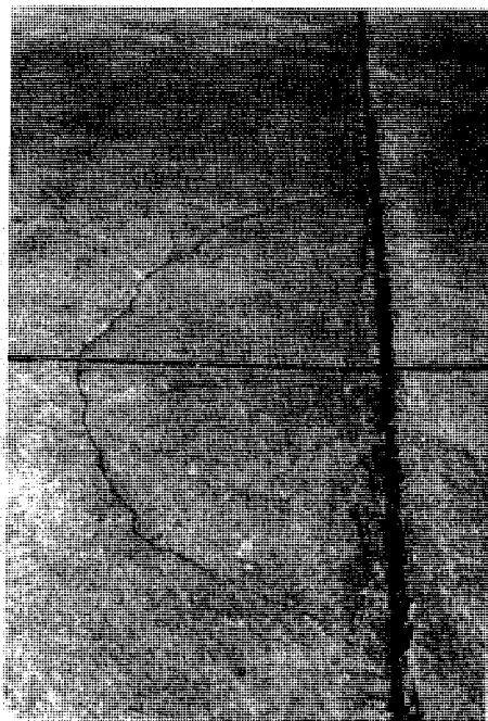
FIG. X2.4 Low-Severity Corner Break
