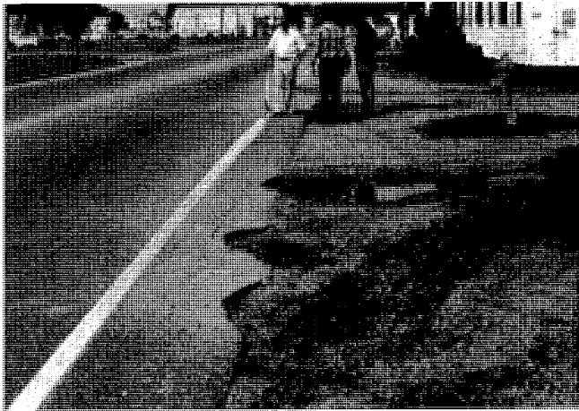
FIG. X1.21 High-Severity Edge Cracking
