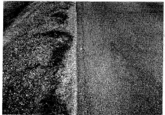
FIG. X1.19 Low-Severity Edge Cracking
