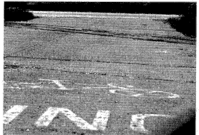
FIG. X2.39 Medium-Severity Railroad Crossing
