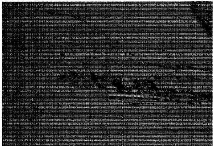
FIG. X1.49 High-Severity Slippage Cracking
