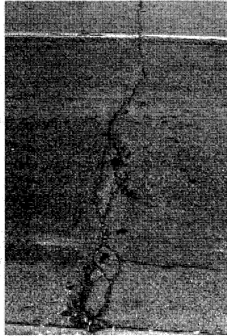
FIG. X1.23 Medium-Severity Joint Reflection Cracking
