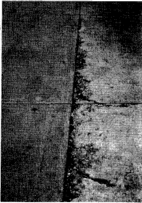
FIG. X2.49 Medium-Severity Spalling, Joint
