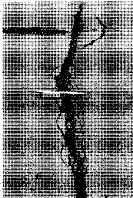
FIG. X1.24 High-Severity Joint Reflection Cracking
