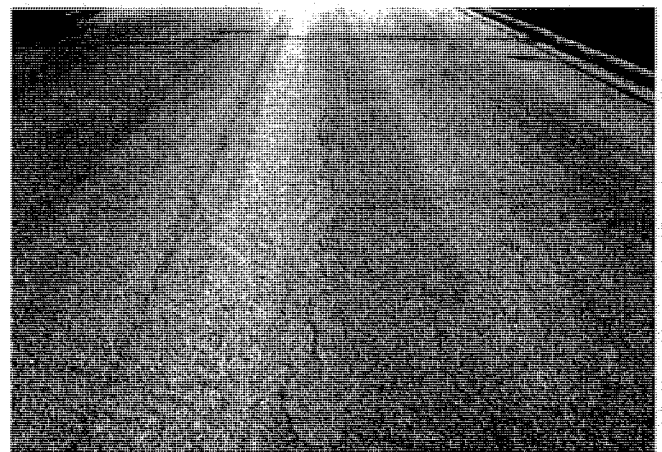
FIG. X1.1 Low-Severity Alligator Cracking
