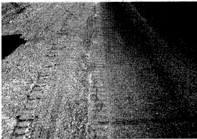
FIG. X1.22 Low-Severity Joint Reflection Cracking
