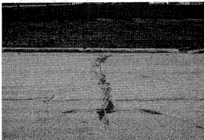
FIG. X1.30 High-Severity Longitudinal and Transverse Cracking
