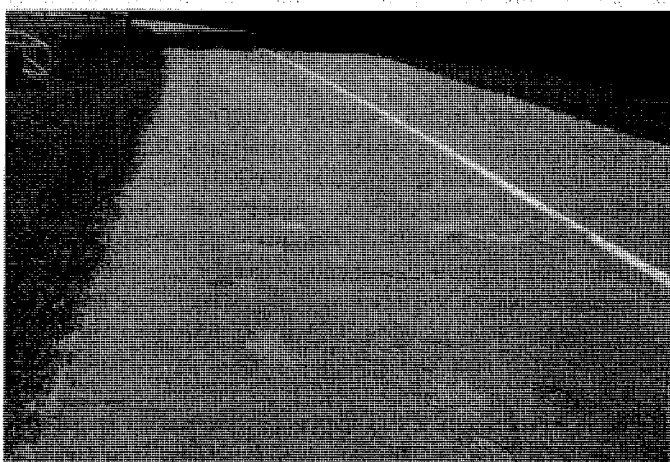
FIG. X1.53 High-Severity Weathering and Raveling
