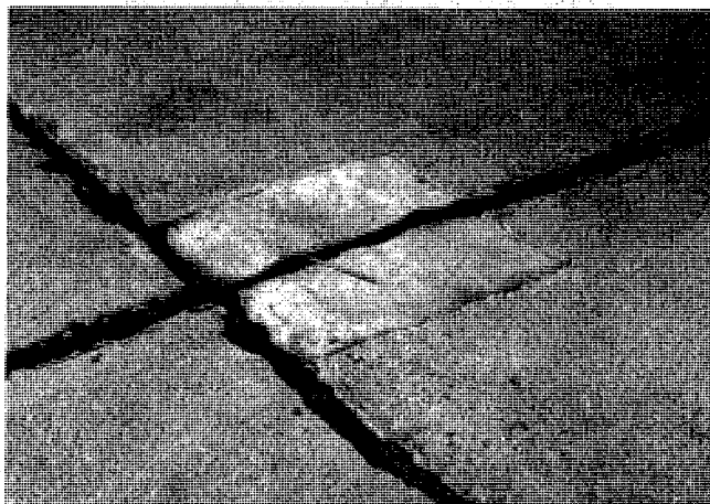
FIG. X2.28 Low-Severity Patching, Small
