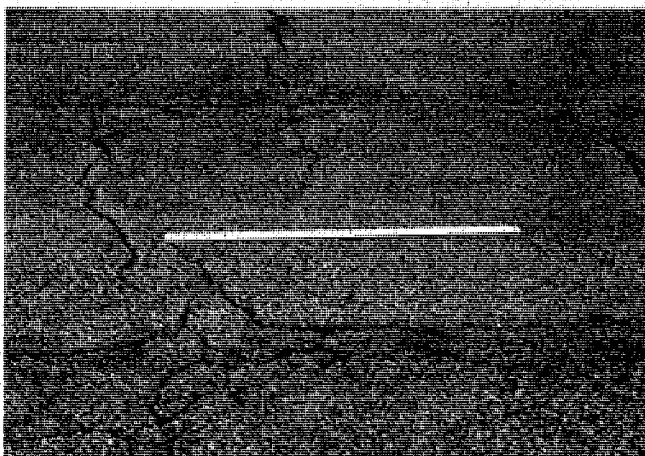
FIG. X1.7 Low-Severity Block Cracking
