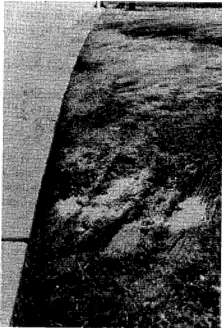
FIG. X2.20 Medium-Severity Lane/Shoulder Drop-Off
