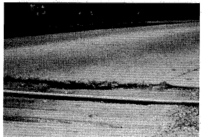
FIG. X2.40 High-Severity Railroad Crossing
