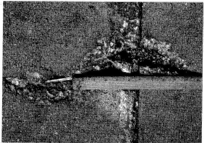
FIG. X2.46 Medium-Severity Spalling, Corner
