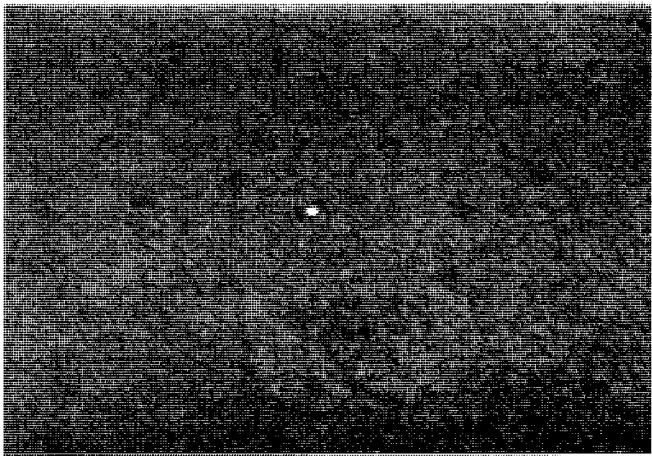
FIG. X2.41 Low-Severity Scaling, Map Cracking, and Crazing
