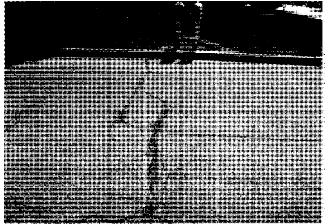
FIG. X1.8 Medium-Severity Block Cracking
